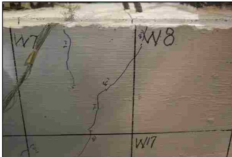
Figure 5.7: EMB80 hairline cracking on the west side of the cap beam at 2.25% drift
