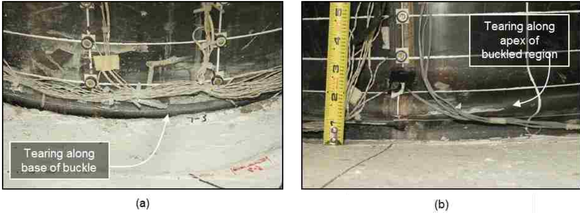
Figure 5.70: EMB96 (a) North and (b) South tube tearing at 8.60% drift South
