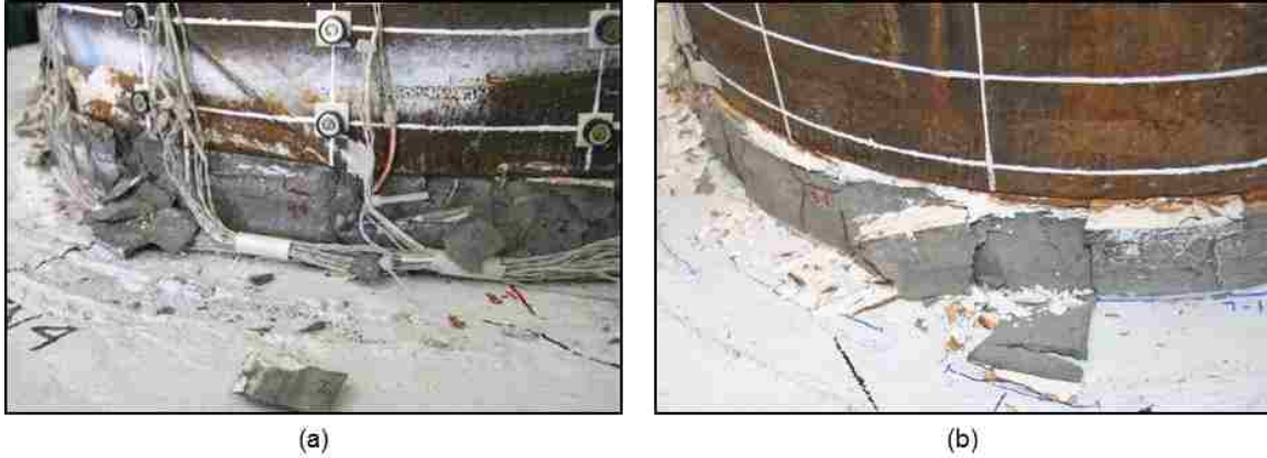
Figure 5.54: WRC Soffit crushing (a) North side of specimen, (b) South side of specimen
