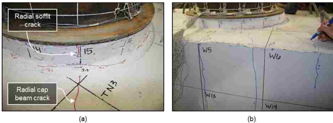
Figure 5.18: WRC radial cracking on (a) North side of column at 1.48% drift, and (b) south side of column at 1.62% drift
