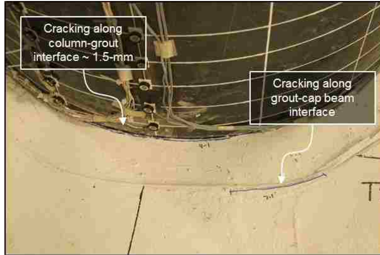
Figure 5.65: EMB96 South grout pad cracking at 1.02% drift North
