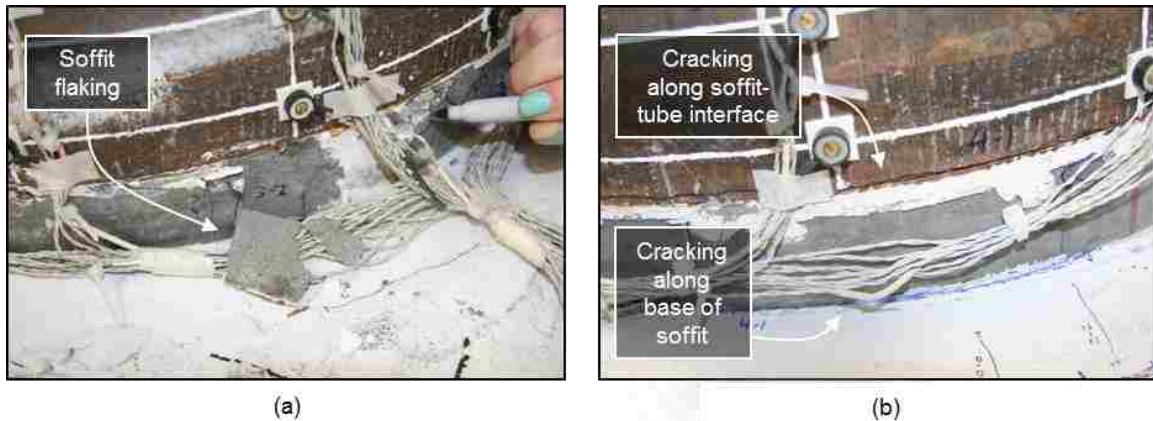
Figure 5.52: WRC (a) Soffit spalling at .28% drift, and (b) Soffit cracking at .44% drift
